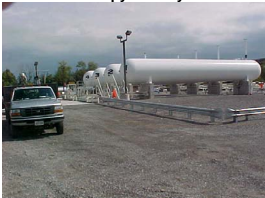
Four new LPG tanks in a high volume cross-border transfer application
