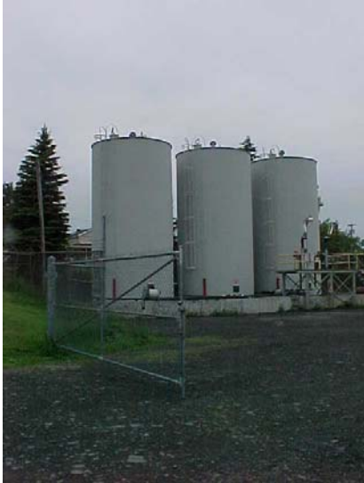
Three vertical #2 fuel oil tanks with signal sent across a public road and at a 40 degree downward angle
