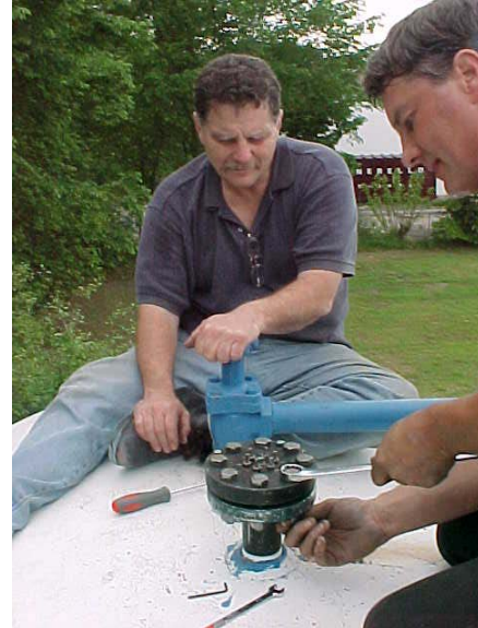
Bill Stehl supervising the install of FTI's patented "pass-through" on a propane gauge.
