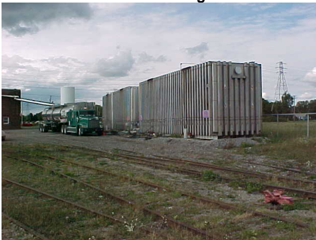
1880 bbl. (70,000 gallon) rectangular tanks for Propylene Glycol
